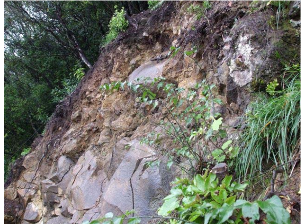
Eroding slope face prior to rockfall netting
