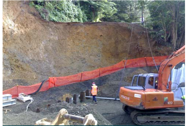
Helena Bay Road Slip
