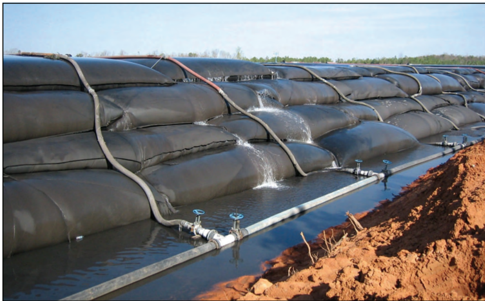
Geotube® technology, perfectly suited to both dewater and contain materials, solved the slurry waste disposal issues facing the North River Mine. This large-scale project involved 3 bag fields, 240 Geotube® containers, and 200,000 cubic yards of coal slurry waste being pumped and dewatered.
