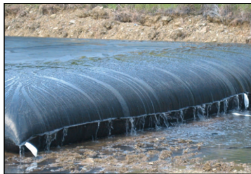
Clear effluent draining during the initial testing phase.
