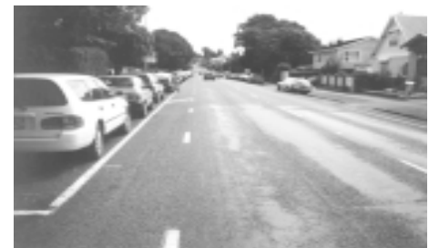
View of Vivian St showing worn surface
