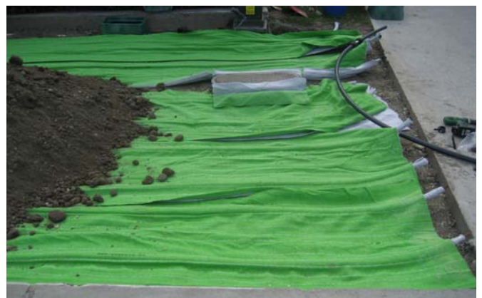
Ready for connection to irrigation system
