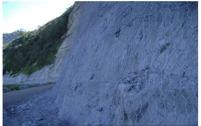
Rockfall netting toe cabling not yet installed against rock face
