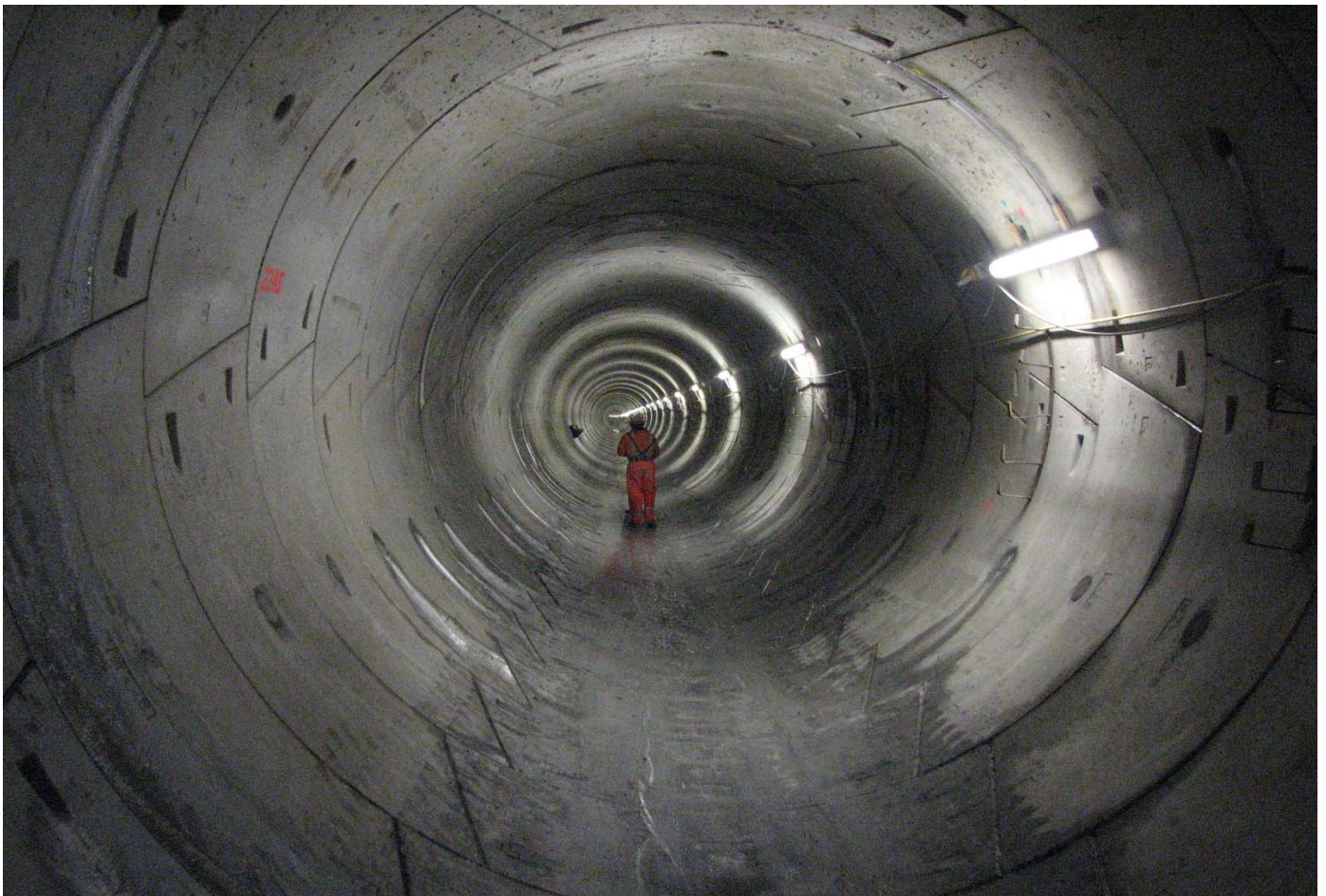
View of the tunnel installed segment lining in the Hobson Bay Tunnel
