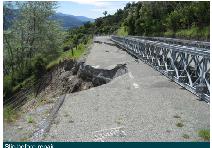
Slip before repair
