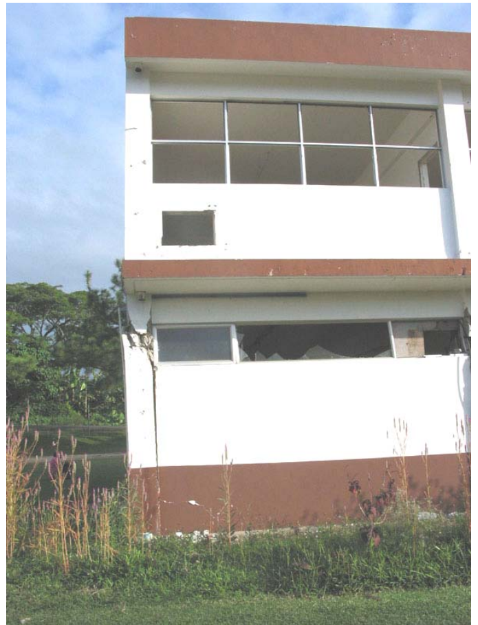
Column damage to school
