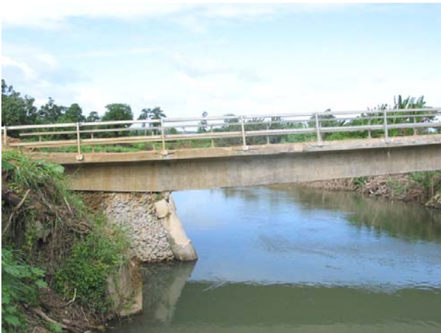
Collapsed bridge pier
